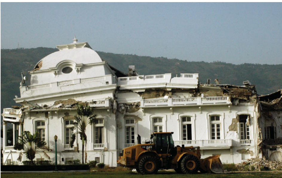
◀ FIGURE 1.2 COLLAPSED BUILDING IN PORT-AU-PRINCE, HAITI A front-end loader is ready for clean-up work in front of the destroyed National Palace in Port-au-Prince, the capital of Haiti. Poor construction of even important government buildings was largely responsible for the great loss of life from the earthquake in 2010. ( St. Felix Evans )
